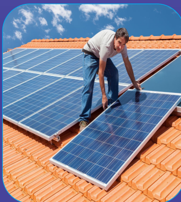
SOLAR ROOF TOP
